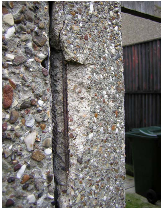
Photograph 3 – Spalling Of Corner Post
